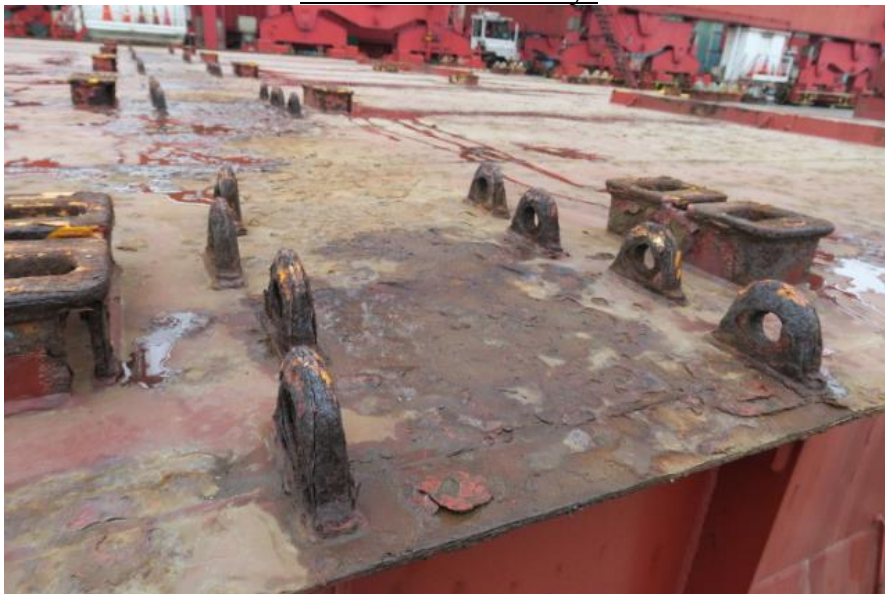
Picture of the same deficiency: Sockets and lashing eyes in cargo area found corroded seriously.
